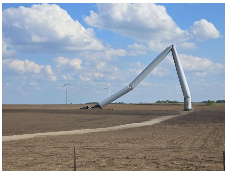
Figure 6. Wind turbine damaged by an F2 tornado near Greenfield, Iowa, May 21, 2024. Source: NWS.
